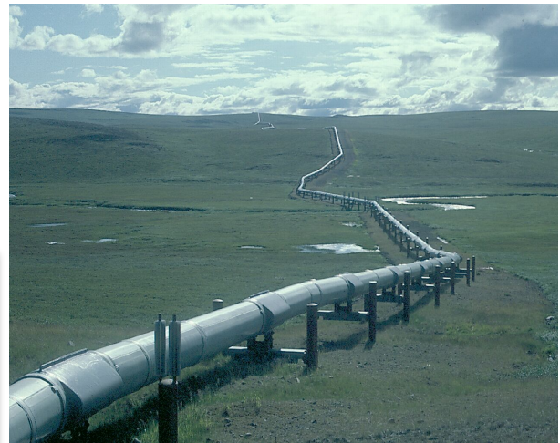
ConocoPhillips deploys DAS-based pipeline monitoring system in Alaska for preventing corrosion-related leakage
